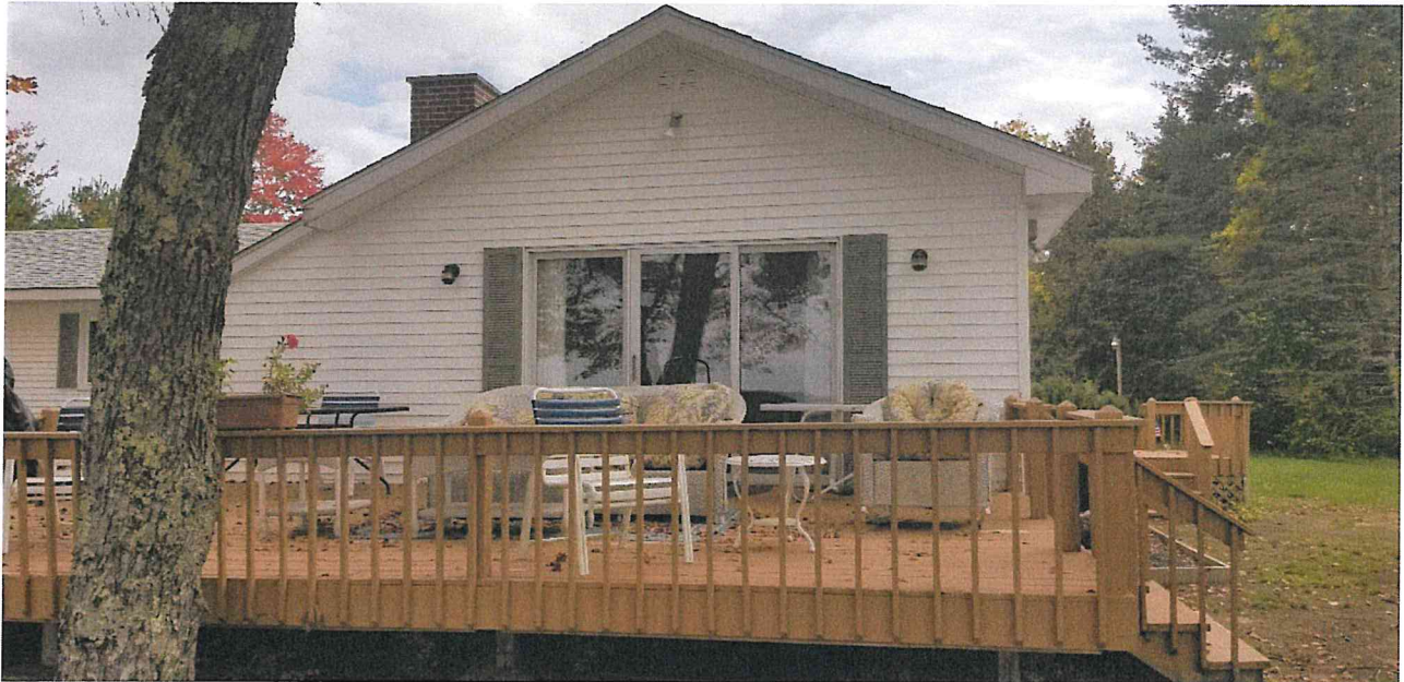
Photo 4: A closer view of the existing deck in front of the camp closer to the shoreline. A smaller deck can be seen to the right side of the building near the back door. It map also be seen in Photo 5.
