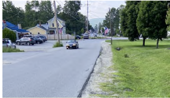
Shoulder erosion on West Road at Village Green
