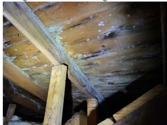
Mold growth on roof sheathing in Attic
