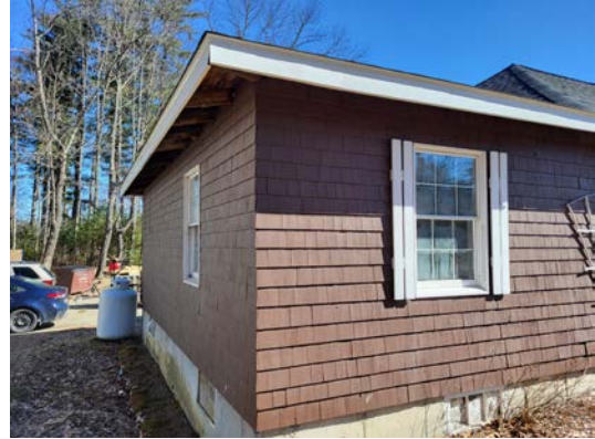
No gutter on this roof line
