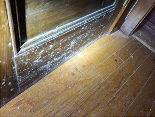
Mold growth on door to Basement
