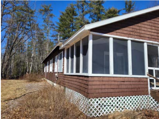
No gutter on this roof line
