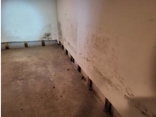
Mold growth on sheetrock in Basement
