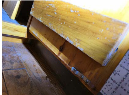
Mold growth on Cabinets
