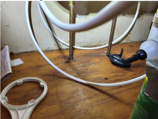
Mold growth on wall in Kitchen sink cabinet
