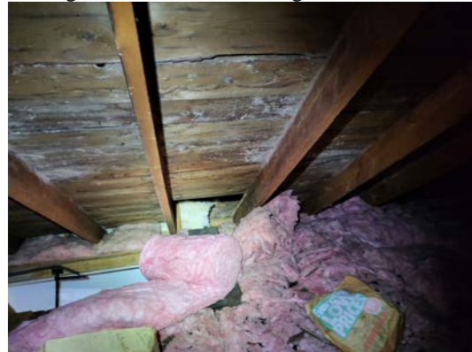
Mold growth on roof sheathing in Attic
