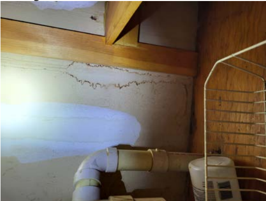
Water damage inside Kitchen sink cabinet
