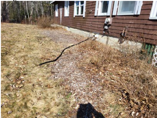
Sump pump discharge
