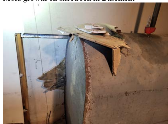
Mold growth on sheetrock fragments in Basement
