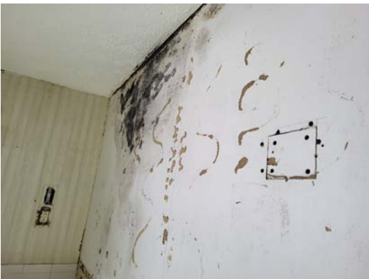
Mold growth on Bathroom wall and ceiling
