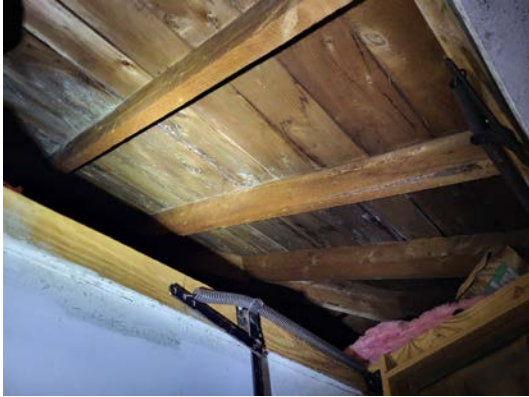
Mold growth on roof sheathing in Attic
