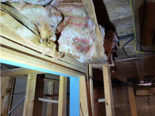
Mold growth on Basement Ceiling insulation
