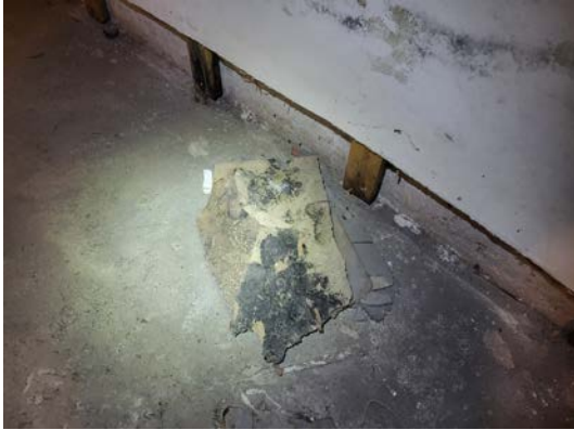
Mold growth on sheetrock fragments in Basement
