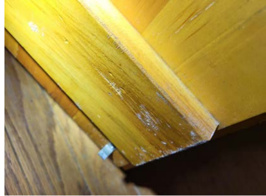
Mold growth on Cabinets
