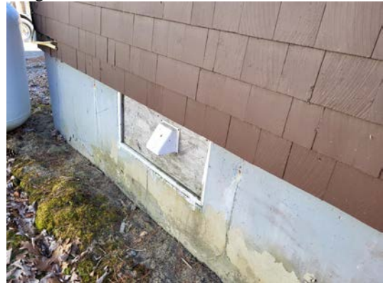
Dryer exhaust outlet
