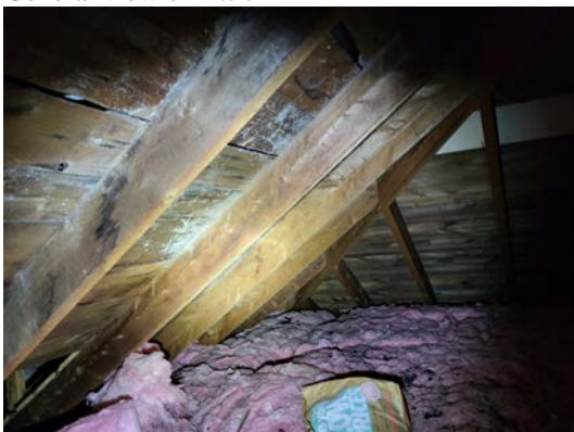
Mold growth on roof sheathing in Attic
