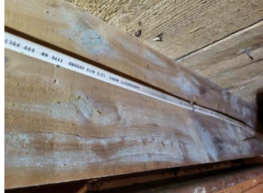
Mold growth on Basement Ceiling
