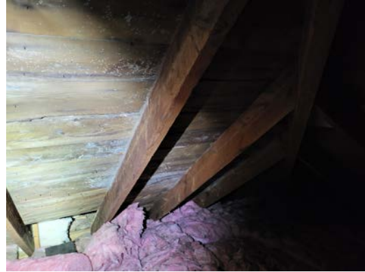
Mold growth on roof sheathing in Attic
