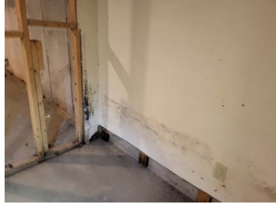
Mold growth on sheetrock in Basement
