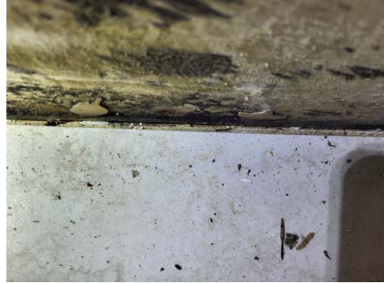
Mold growth appears to extend onto sub-floor in Bathroom
