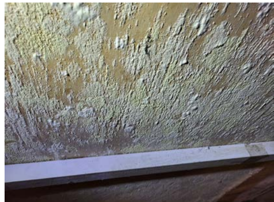
Significant mold growth on door to Bulk-head
