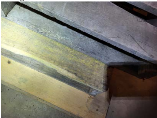
Mold growth on pallets in Basement
