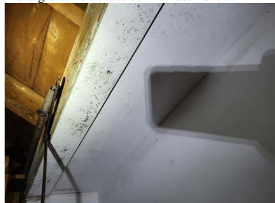
Mold growth on Ceiling in Stairwell to Basement
