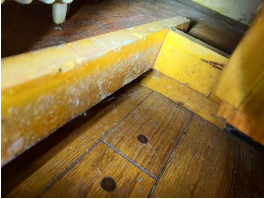
Mold growth on Cabinets
