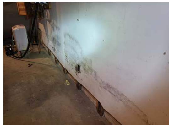
Mold growth on sheetrock in Basement
