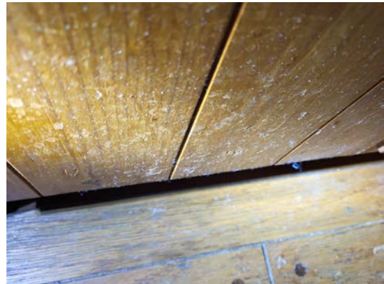
Mold growth on Cabinets
