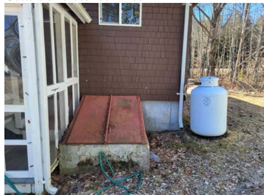
Gutter downspouts deposit water along foundation
