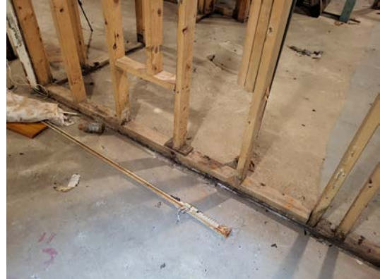
Mold growth on wall framing in Basement
