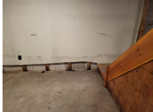
Mold growth on wall framing and sheetrock in Basement
