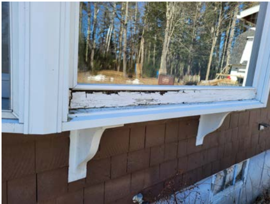
Picture Window frame is degraded
