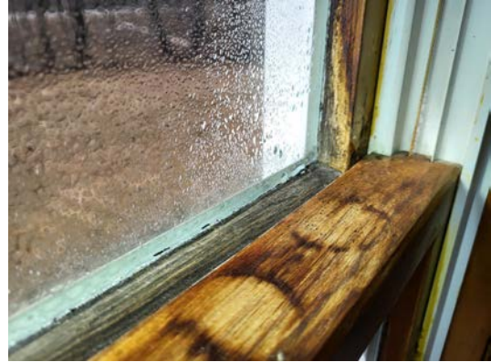
Example of condensation on windows and mold on window sashes
