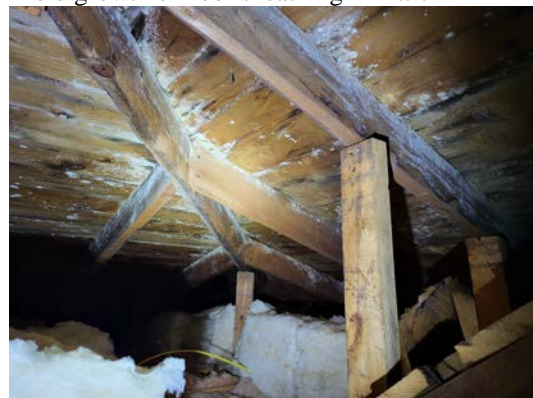
Mold growth on roof sheathing in Attic
